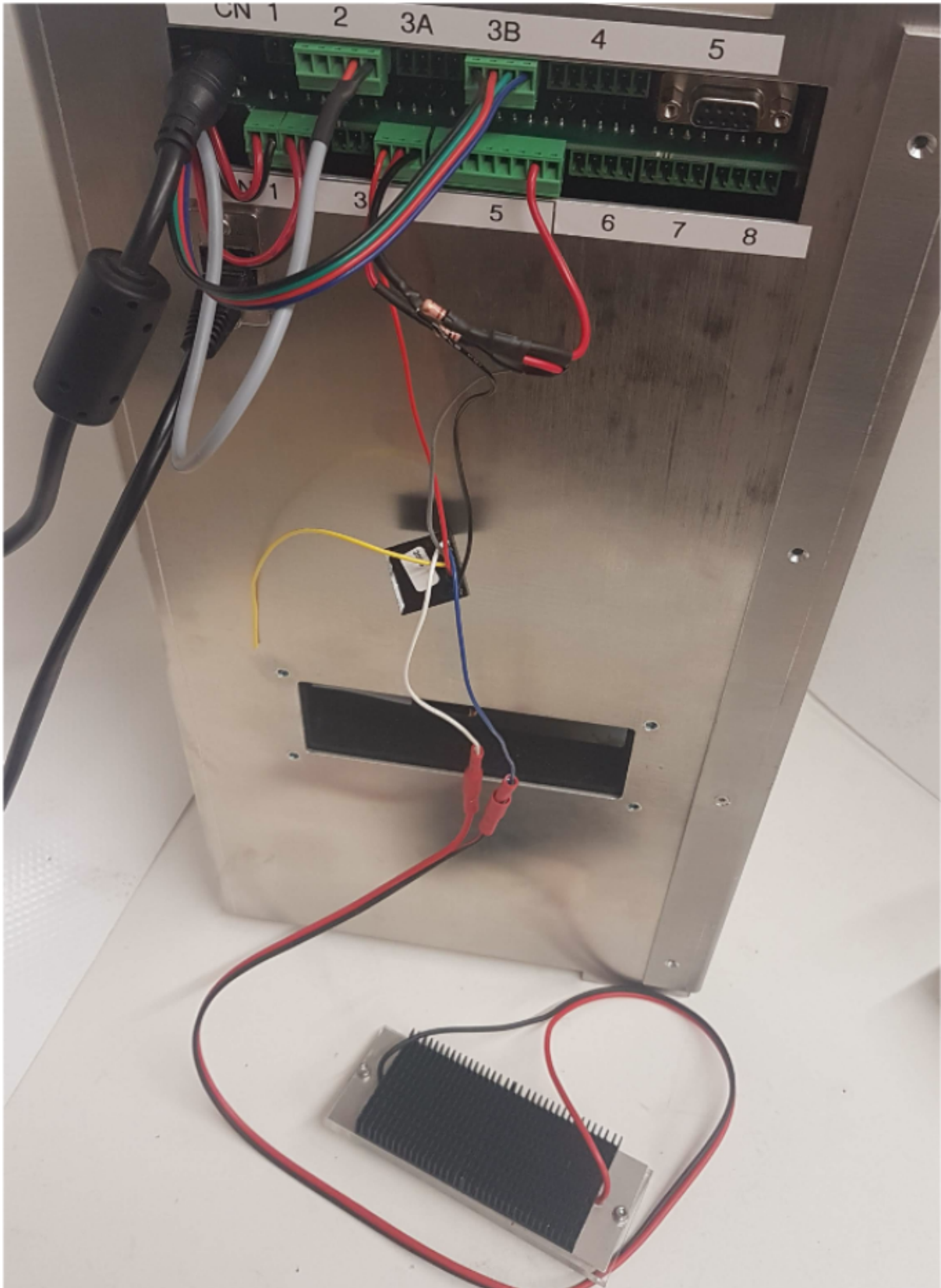
Connection of the LED holder to the MWP unit via the control circuit
